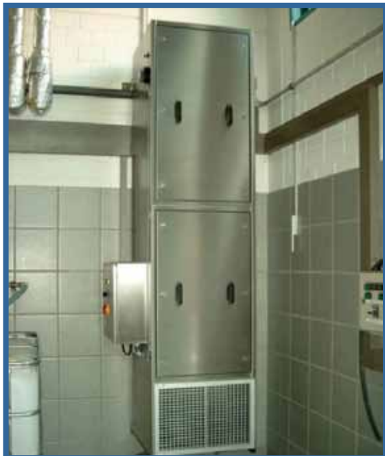
Dewatering Room 2,400 cfm
