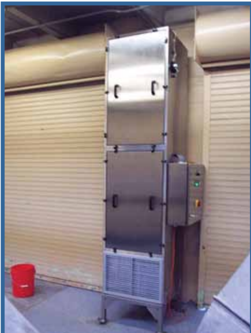
Headworks in Evergreen, CO 2500 cfm
