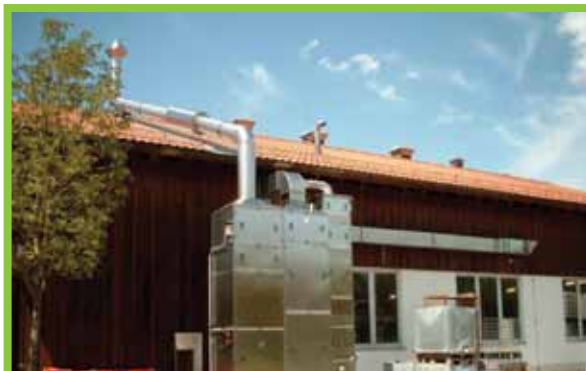
Sludge Dryer - 1200 cfm
