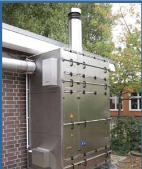
Pump Station. Velton PS 2008
